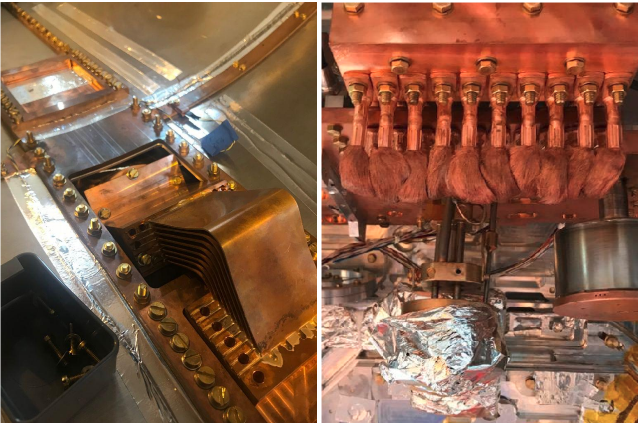
Figure 5.45: Differences between the first design of the thermal link coming from the PT cold head to the 4 K shield. On the left: the first design mad with different stacked copper plate, this have been modified with 10 copper braids for an optimized thermal link ( right )
