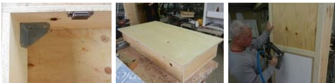
Figure 67. Pictures during the production of the GDC wall prototype. From left to right: 1. Wooden box with connection triangle and magnet for the top, 2. Wooden box completed, 3. Fixing foil and the box with wooden slats connected with the intermediary wooden slats. (photo Androšević)
