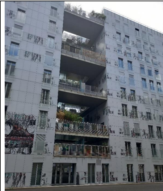
Figure 122 E5 building, Fault, north façade. Source M. Apostolou
