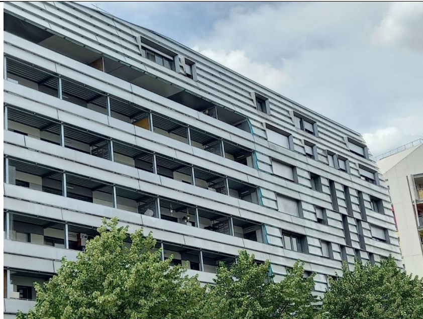
Figure 63 The main facade of the building is, in fact, a cladding in extruded polycarbonate, made with inclined panels arranged in tiles. Source M. Apostolou
