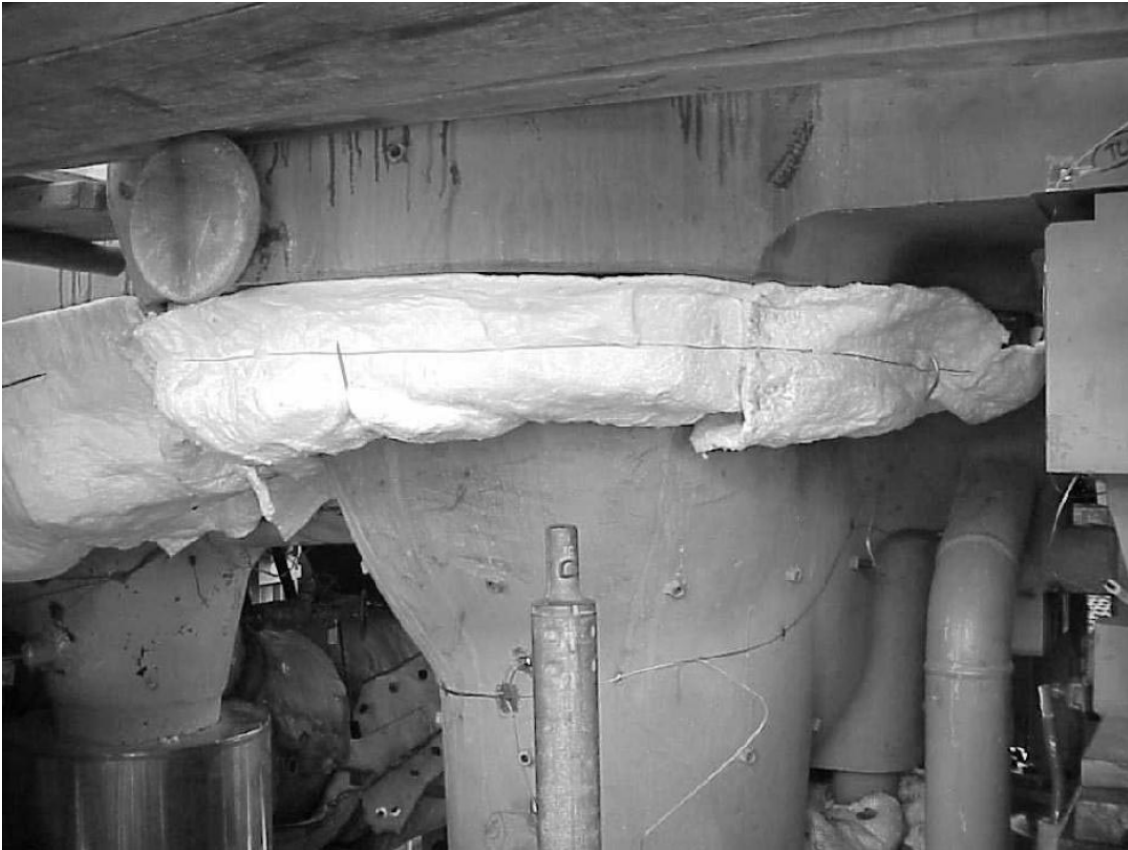
Photo 3 - Bottom portion of the horizontal joint. (Cold reheat part of the turbine with nuts covered.)
