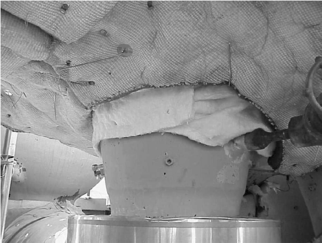
Photo 6 - Bottom of the turbine. Intersection of the main steam inlet and hot reheat shall be covered with 1/4 inch to 1/2 inch thickness of insulation before installation of inner layer.
