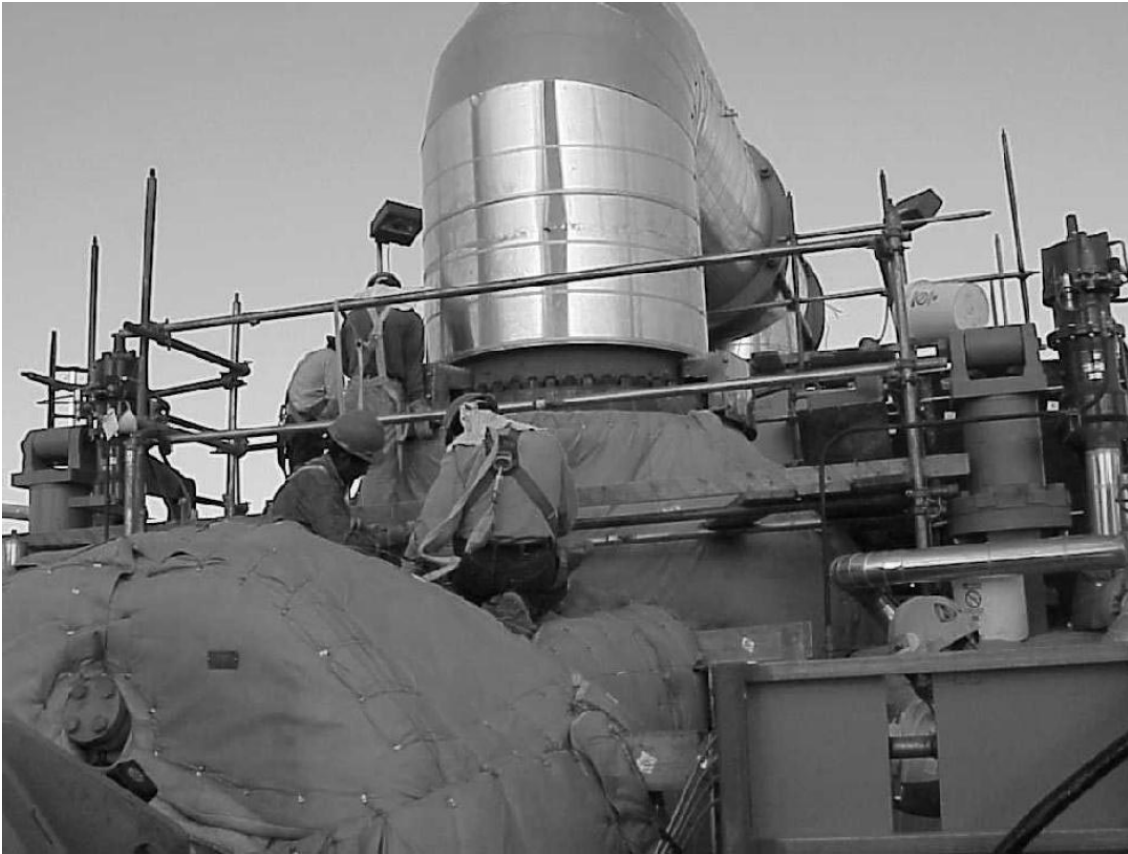
Photo 10 - View of the turbine with outer layer blankets installed. Installation of the removable metal cover for HP/IP crossover. Borescope opening has not yet been covered with blanket installation.
