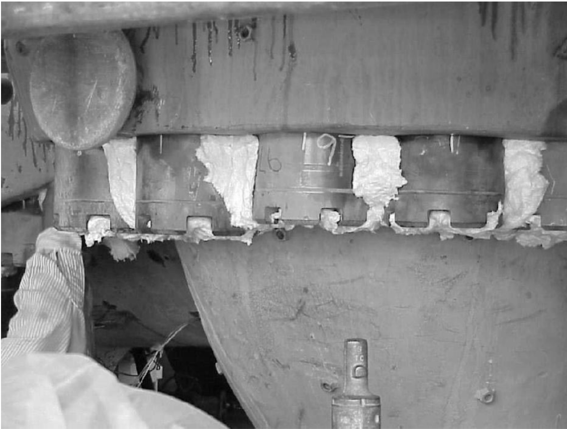
Photo 1 - Bottom part of the horizontal joint of the turbine. Stuffing insulation (scrap) between and behind nuts.
