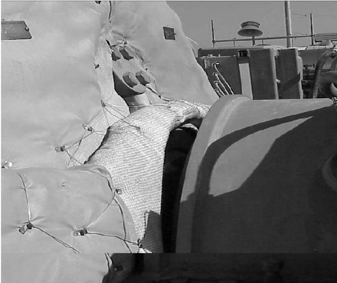
Photo 13 - View of the air gap between front bearing housing and turbine blankets.
