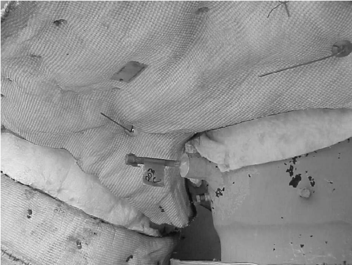
Photo 5 - Bottom of the turbine. Intersection of the main steam inlet and hot reheat with inner layer blankets only. Quantity of studs with nails for the bottom of the turbine should be determined to prevent sagging of blankets. Blankets shall be installed without any gaps.
