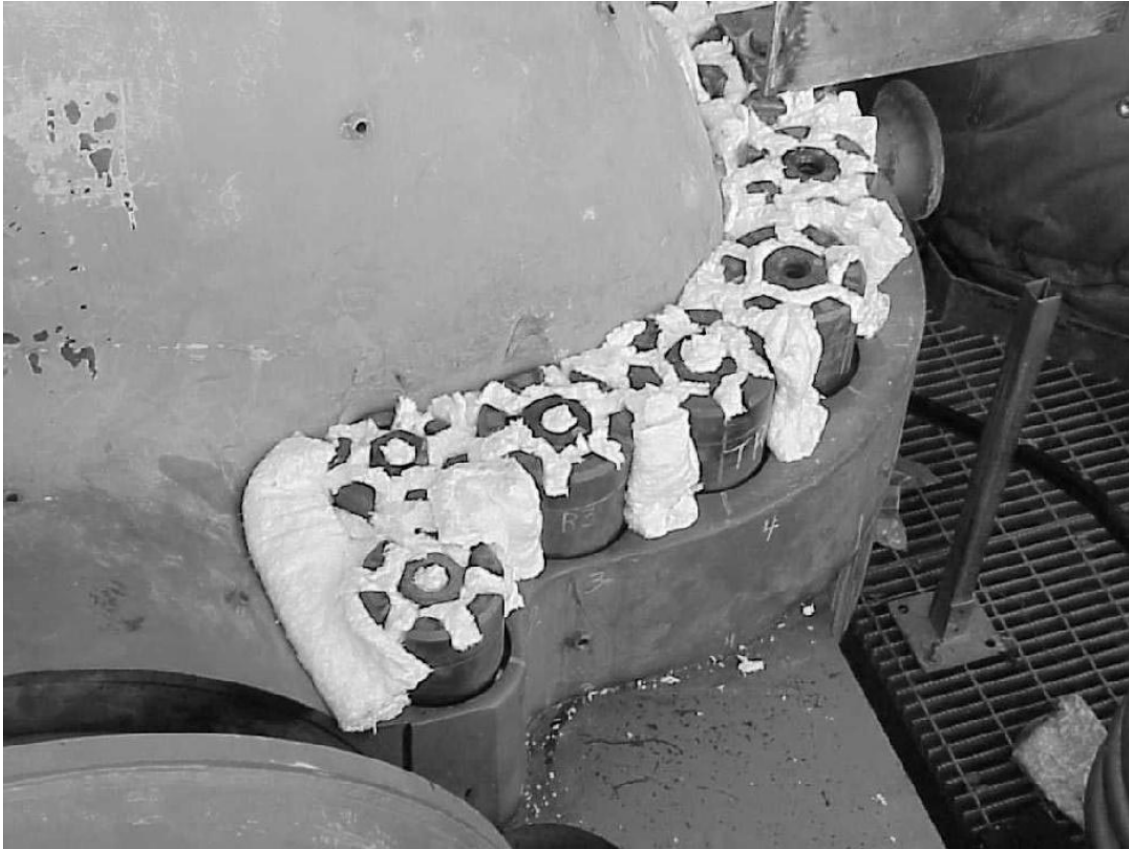
Photo 2 - Top portion of the horizontal joint of the turbines. (Stuffing of the insulation.)
