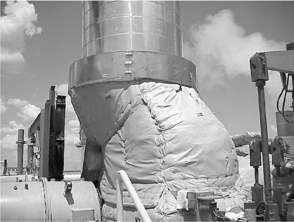
Photo 11 - Back side of the turbine with assembled removable blankets at crossover connection.
